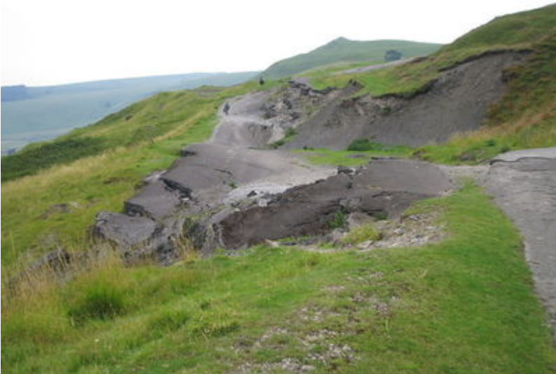
The Mam Tor landslide: the Turn Pike Road damaged by the landslide.
